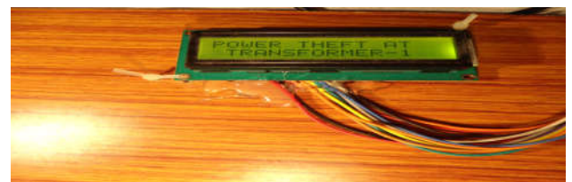
Fig 7 Display in LCD at the substation when theft is done along with alarm
